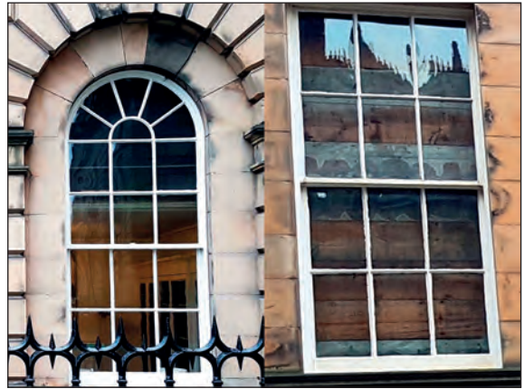
Fig. 7. Left, supporting structure for an upper floor crosses ground floor window. Right, fully furnished window on first floor boarded up on the inside. Author photos
